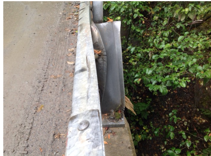
damaged steel posts
